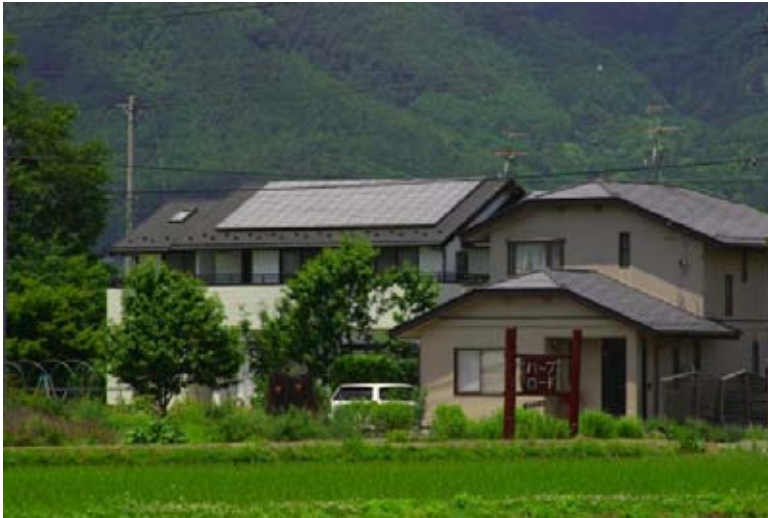
Photo voltaic grid feedback electric power array on rural house in Nagano prefecture
